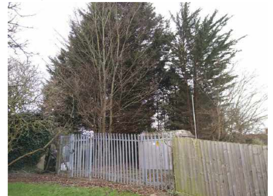
10. Sub-Station adjacent to site with access required
